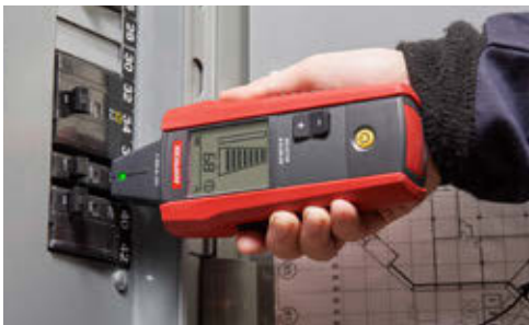
Identify the single correct breaker
