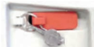
Locked with Wire Seal
